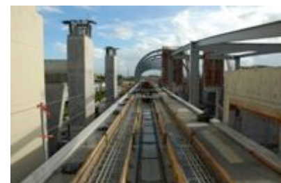
Heavy Rail Electrical Isolation
