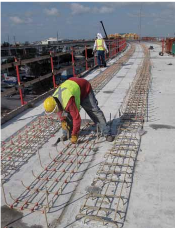
Fig. 5: A worker prepares to trim the legs of a plinth cage to set the correct height before installing it over the projections of the plinth stirrups (to his left). To the worker's right, bar cages have been installed over the stirrups in the guideway deck
