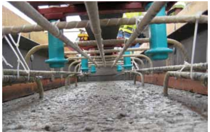
Fig. 6: Plinth stirrups, cages, and rail fastener anchor inserts (blue) prior to concrete placement
