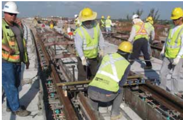
Fig. 3: The trackwork contractor was responsible for installing the plinth reinforcing, setting the rails, and placing the concrete within plinths and pedestals. Here, workers are positioning rail anchors and assembling plinth forms. The GFRP plinth reinforcing and insulated rail anchor inserts can be seen below the rails
