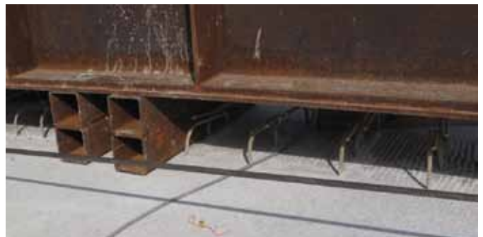
Fig. 7: Gantry cranes and other equipment sometimes conflicted with GFRP bars. Here, the bars at a reaction point for a crane girder have been trimmed flush with the deck. They will be replaced before completion of the rail plinth
