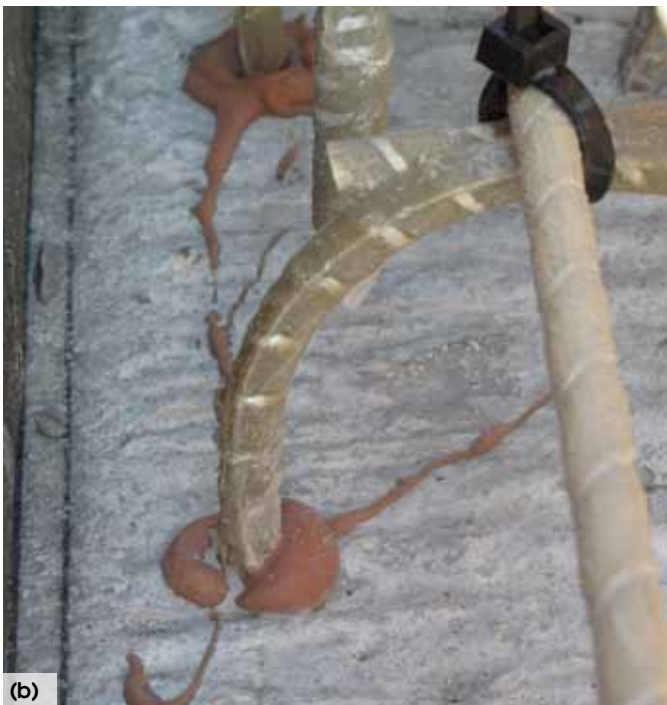
Fig. 8: If damaged, GFRP bars could be replaced with new bars anchored using epoxy adhesive: (a) damaged bars have been marked for replacement; and (b) after the existing bars were cut off, new bars were installed in holes drilled through the existing bar
