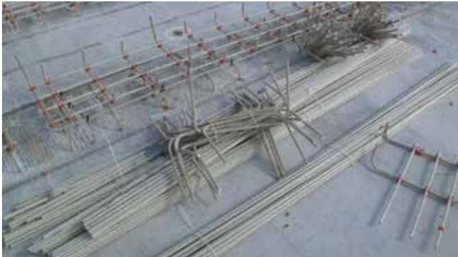
Fig. 4: GFRP bar kits comprised hooked and straight bars for the trackwork contractor to assemble into plinth cages as required
