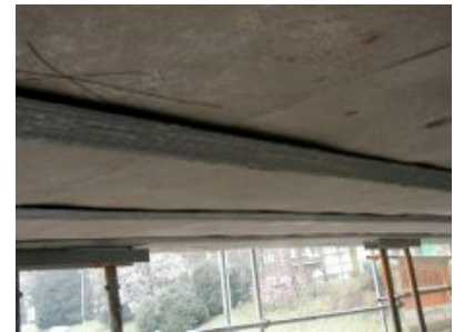
Inadequate surface leveling !
